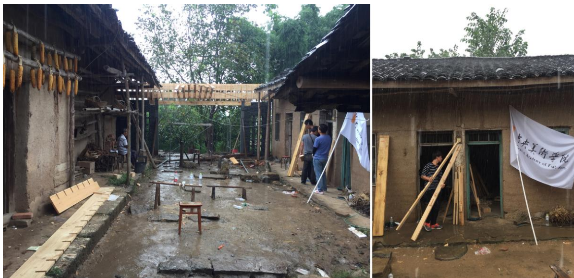
Figure 7. The heavy rain slowed down construction, The team sorted out materials in rainstorm Source by author [2017]
