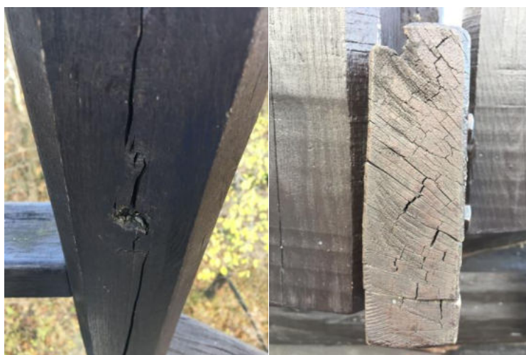
Figure 10: Cracks in the Makovecz Imre lookout tower
