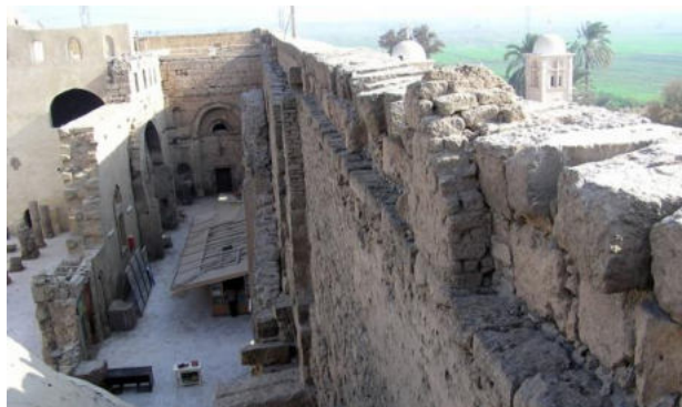
Fig. 8: Exterior walls of the White Monastery – Gabra Gawdat, Gertrud J.M., Van Loon
