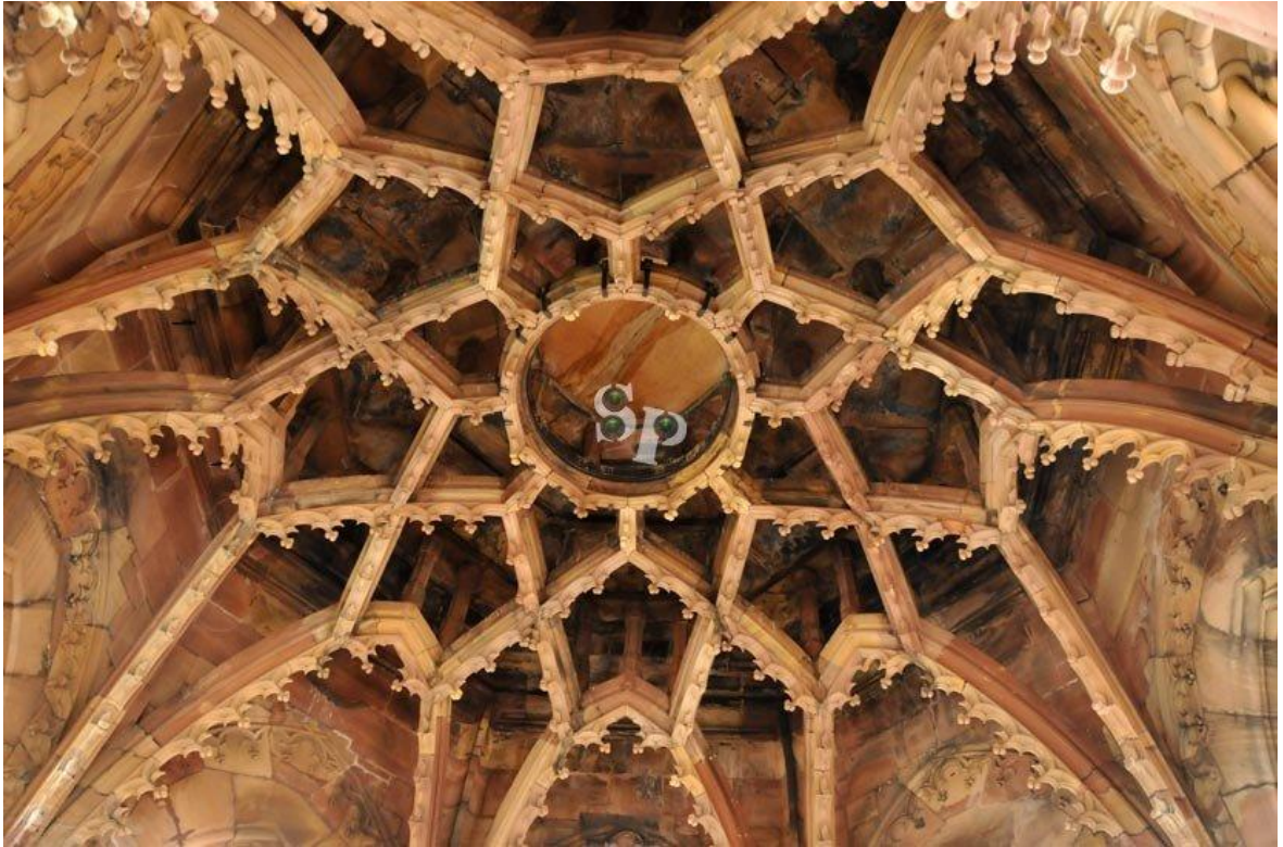
Image 6 The vault of the tower octagon. Photo by Patrick Boehler. Source: http://www.strasbourgphoto.com/la-fleche-de-la-cathedrale/#!sxb-[g5056]/0/
